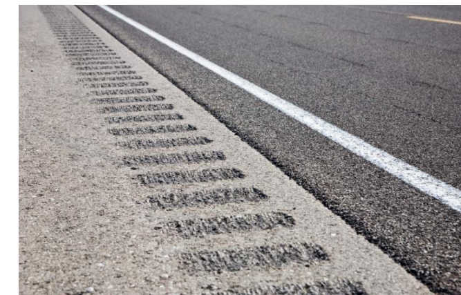
Figure F-21: Rumble Strips
